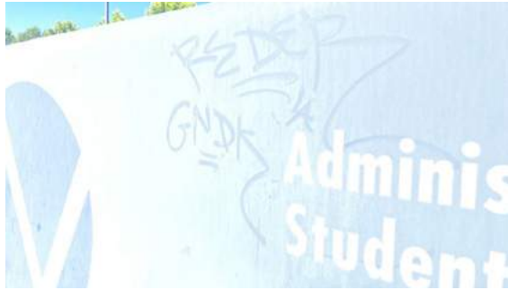
RESIDUE AND VANDALISM
