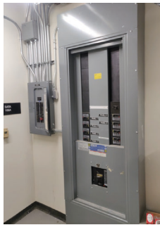
North Complex Electrical Room
