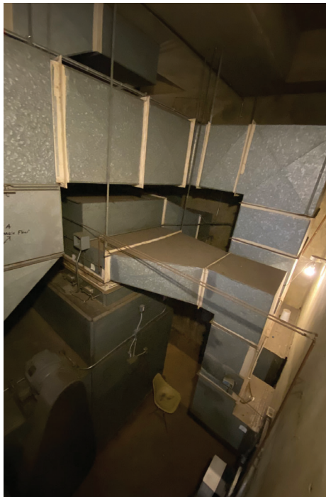
Multi-Zone unit at Crafton Hall
