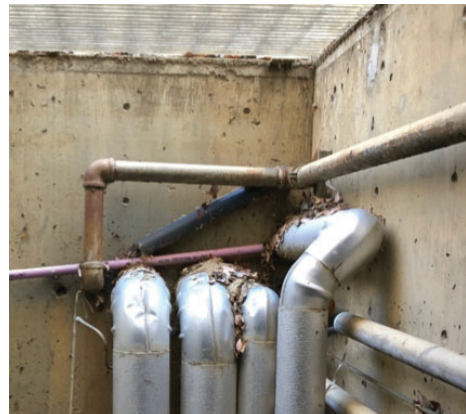
2" gas line entering Central Complex 2 below grade
