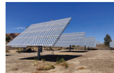
Solar Field PV Panels
