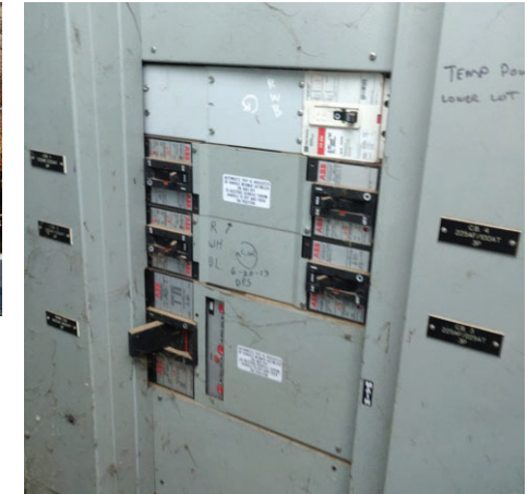
CDC Main Switchboard
