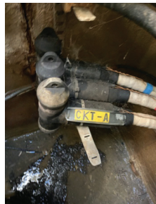
T-body Splice in Manhole
