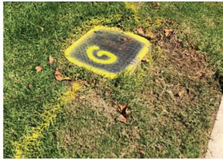
Gas vault along campus drive, south of the gym building
