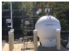
Compressed natural gas filling station
