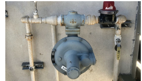
Gas meter, GPR and EQV serving the rooftop equipment of KHA building
