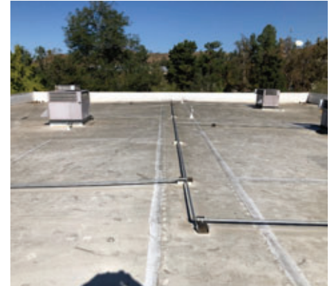
Gas piping serving the rooftop equipment of East Complex 2
