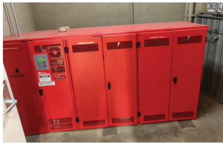
Performing Arts Uninterruptible Power Supply
