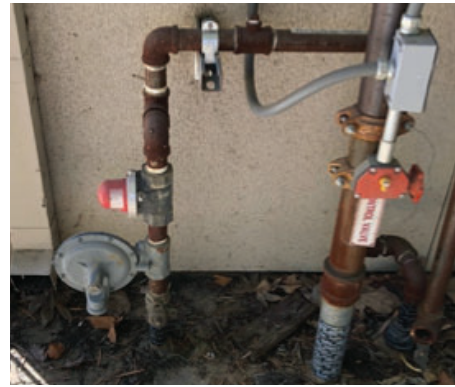
1-1/4” gas line serving the North Complex buildings
