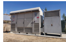
Solar Field Electrical Yard
