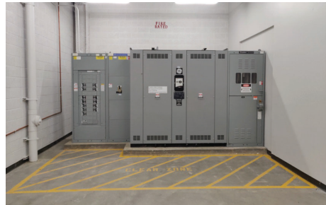
Public Safety and Health Sciences Unit Substation
