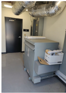
North Complex Electrical Room
