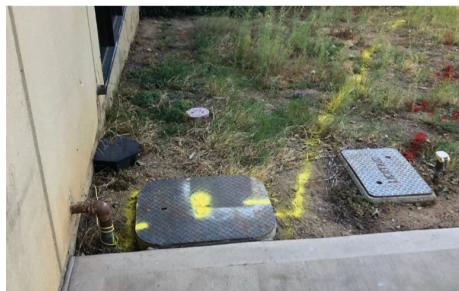
1-1/4" gas line entering Visual Arts building
