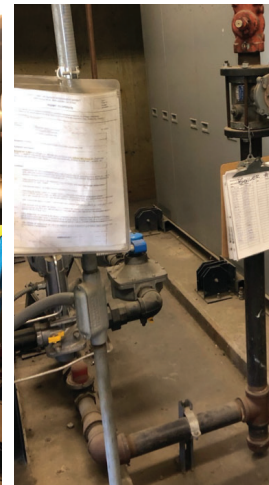
Gas feed to boiler with gas meter, GPR, and EQV
