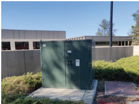
Parking Lot I Selector Switch HVS-I
