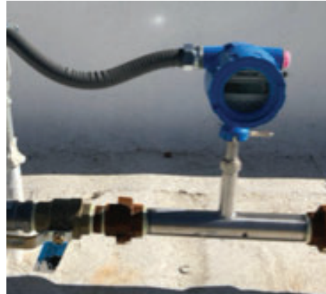
Gas meter on the roof of East Complex 1
