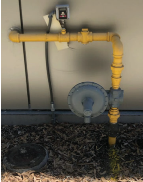
Gas feed serving the east side of the Crafton Center
