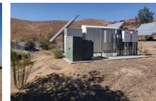
Solar Field Electrical Yard
