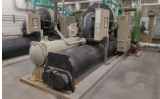
Central Plant Chiller
