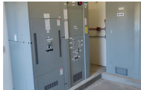
Crafter Center Main Switchboard
