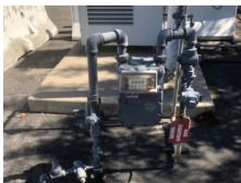
Gas meter serving compressed natural gas filling station
