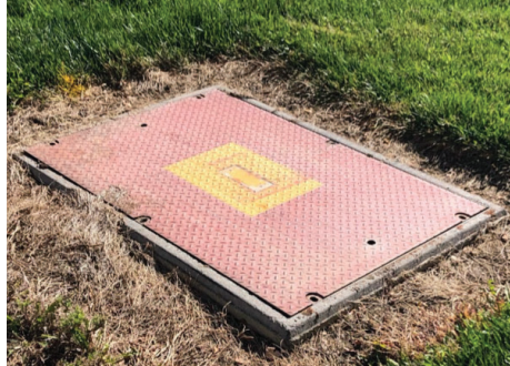
Gas vault on located to the east of the Learning Resource Center
