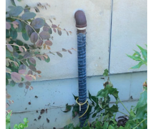
1-1/2" gas line entering East Complex 2
