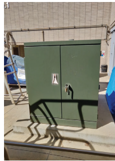
Aquatics Complex Outdoor Padmount Transformer
