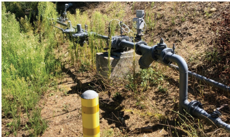
Main campus gas meter assembly located east of lot M"
