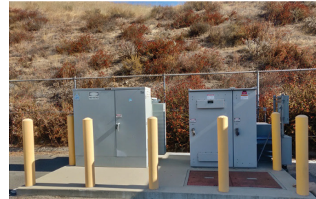
M&O Facility Outdoor Padmount Transformer and Main Switchboard
