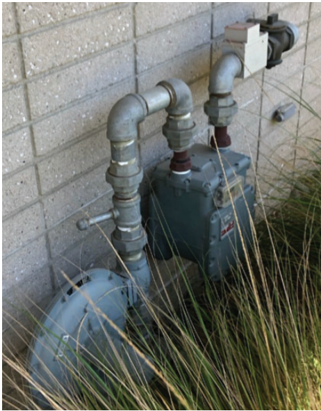
2” gas line entering the Public Safety and Allied Health building
