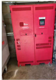
Aquatics Complex Uninterruptible Power Supply
