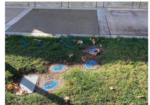
CHW and HHW Valves
