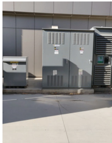
Canyon Hall Electrical Yard
