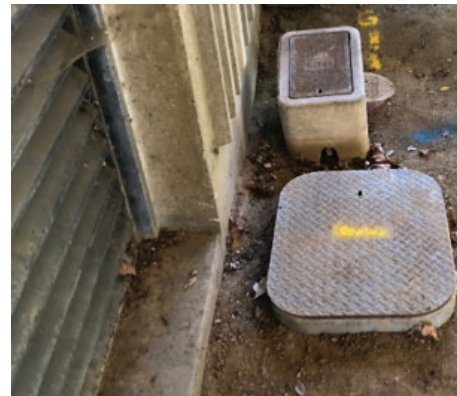
3/4" gas feed serving the east side of Crafton Hall
