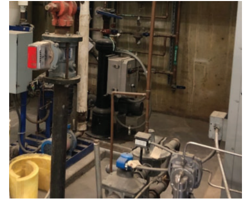
Gas feed to boiler with gas meter
