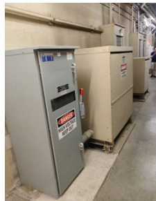
Performing Arts Dry Type Transformer and Load Interrupter Switch
