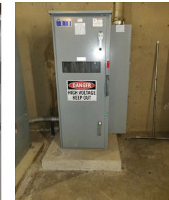
Chemical Health Sciences Load Interrupter Switch
