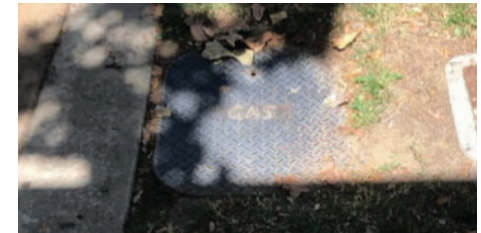
Gas vault north of the Central Complex 1 south wing
