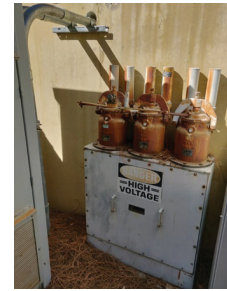
Gymnasium Complex Oil Switch
