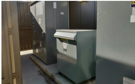
Canyon Hall Unit Electrical Yard
