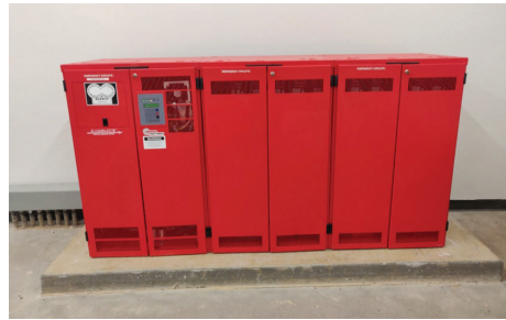
Public Safety and Health Sciences Uninterruptible Power Supply
