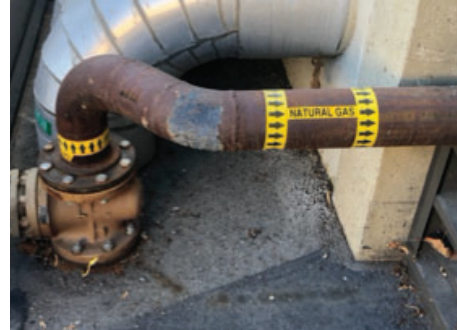
Main 6" gas feed serving the Central Complex 1
