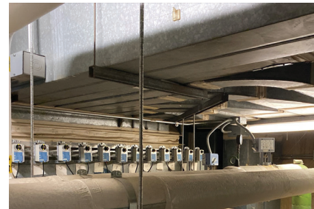
Zone damper actuators on Multi-Zone at West Complex building
