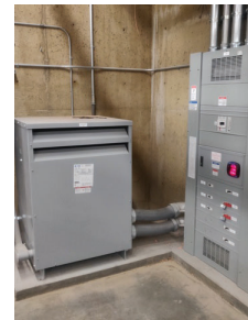
LADM Electrical Room
