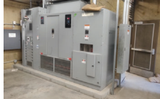
Central Plant Unit Substation
