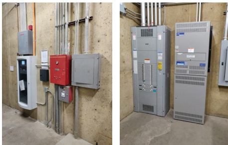
Student Services Administration Electrical Room
