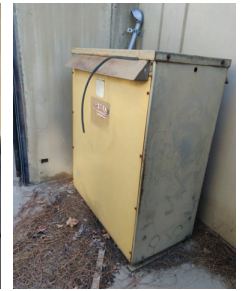
Gymnasium Complex Dry Type Transformer
