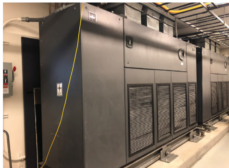
Computer Room Air Conditioning (CRAC) units at Learning Resource Center
