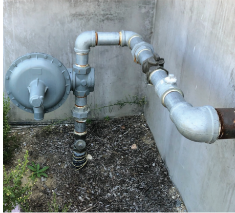
3" gas line entering Canyon Hall
