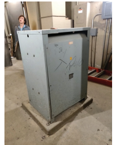
Chemical Health Sciences Electrical Room
