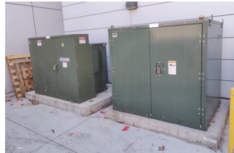
Crafter Center Outdoor Padmount Transformer and Selector Switch
