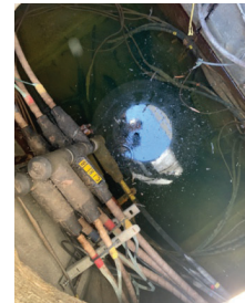
T-body Splice in Manhole
