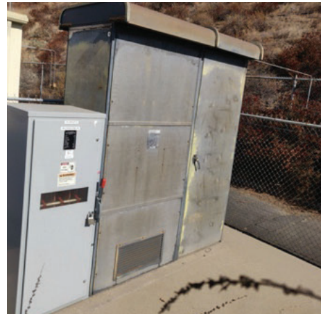
M&O Facility Outdoor Dry type Transformer and Load Interrupter Switch
