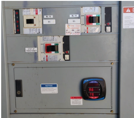
Visual Arts Main Switchboard
