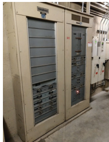
Performing Arts Main Switchboard
