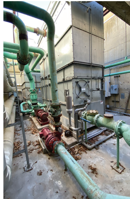
Cooling Towers and CW Pumps at Central Plant
