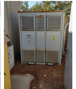
Gymnasium Complex Dry Type Transformer
