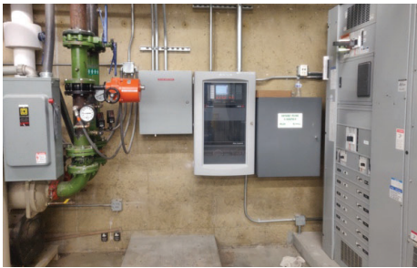
Central Plant Electrical Room
