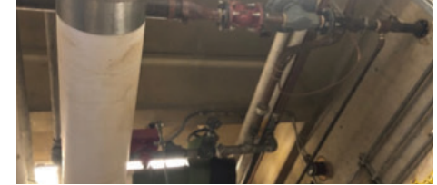
Gas feed with GPR entering to serve the rest of the Central Complex 1 building
