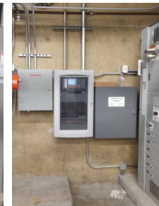
LADM Electrical Room
