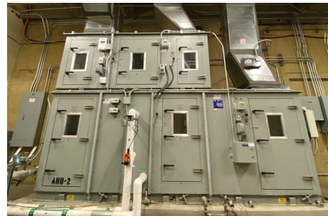
AHU at Clock Tower Building
