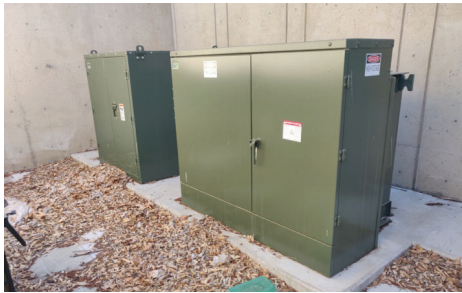
LADM Building Outdoor Padmount Transformer and Selector Switch HVS-A
