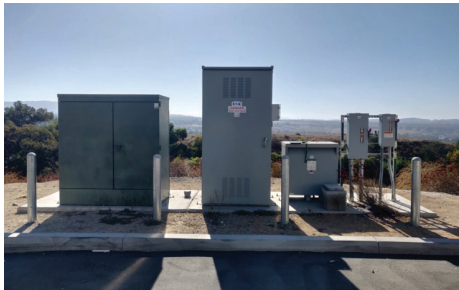
Visual Arts Electrical Yard
