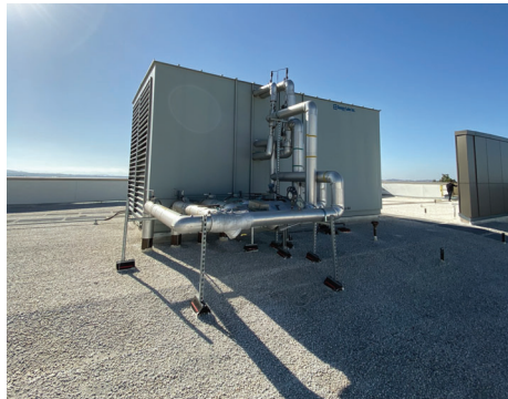
AHU on Canyon Hall Roof
