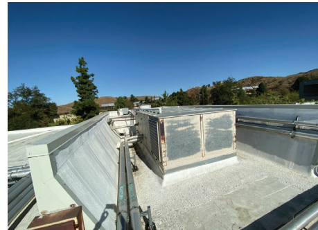
Multi-zone unit on Visual Arts building roof
