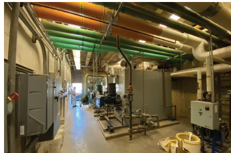
Boilers in Central Heating Plant at Central Complex 1
