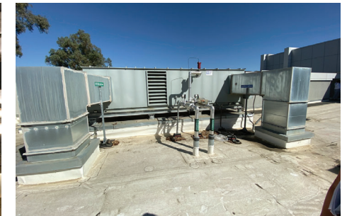
Air handling unit on Crafton Center roof
