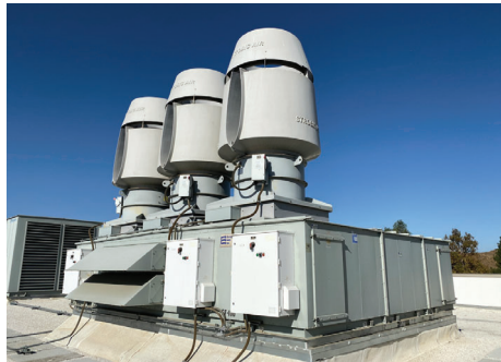
Laboratory Exhaust Fans on Canyon Hall roof
