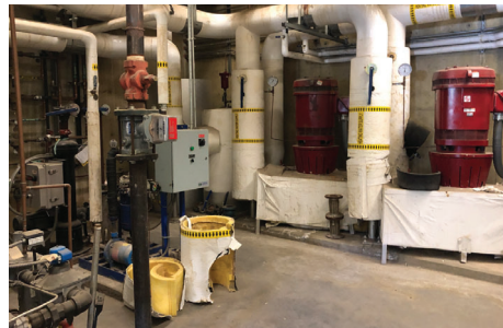
HHW Pumps in Central Heating Plant
