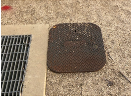
Gas vault north of Central Complex 2
