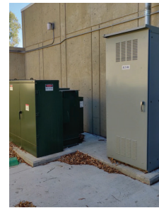
LADM Electrical Yard
