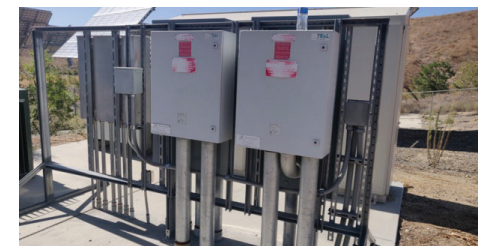
Solar Farm Inverters
