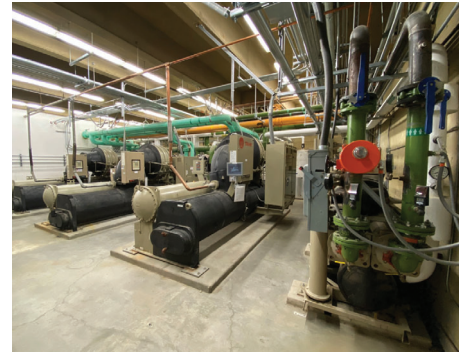
Chillers at Central Plant
