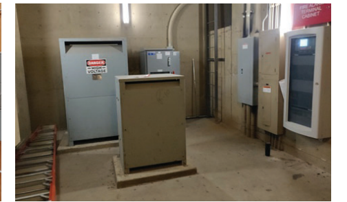
Chemical Health Sciences Electrical Room
