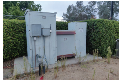
CDC Outdoor Substation
