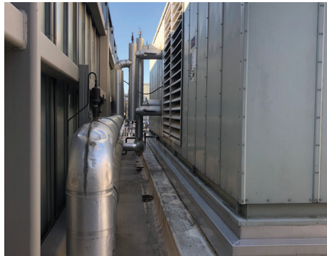
CHWSR and HHWSR connections AHU on Learning Resource Center Roof
