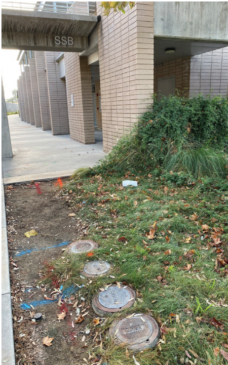
CHW and HHW Valves
