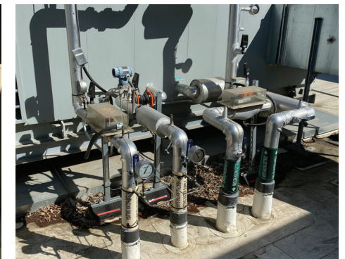
CHWSR and HWSR connections to AHU at Crafton Center
