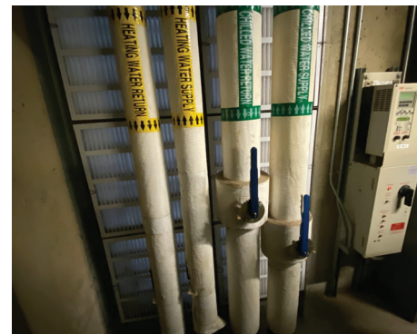
CHWSR and HWSR lines at West Complex Building
