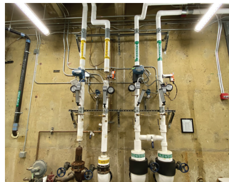
CHWSR and HWSR lines at Clock Tower Building
