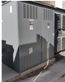
Canyon Hall Unit Substation
