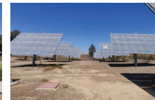
Solar Field PV Panels
