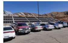
Solar Field PV Panels
