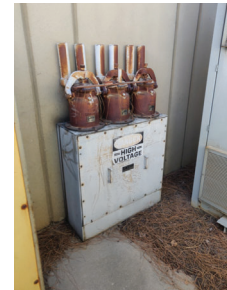
Gymnasium Complex Oil Switch
