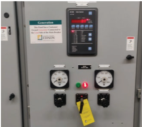
Main Switchgear Meter and Switches
