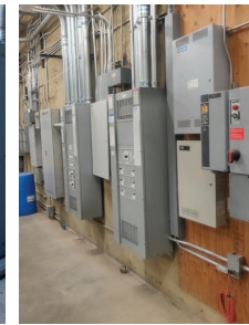
LADM Electrical Room
