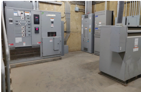
Student Services Administration Indoor Unit Substation
