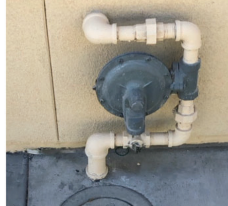
1-1/2" gas line entering East Complex 1
