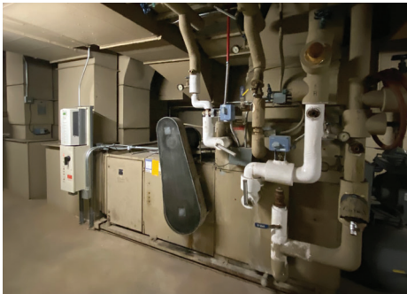
Multi-zone unit in Central Complex 2
