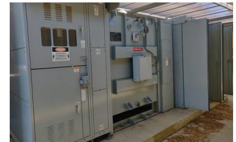
LRC Unit Substation
