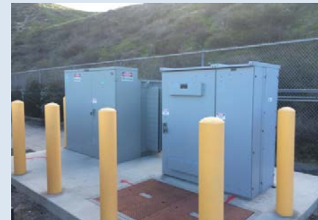
Walking electrical switch gears
