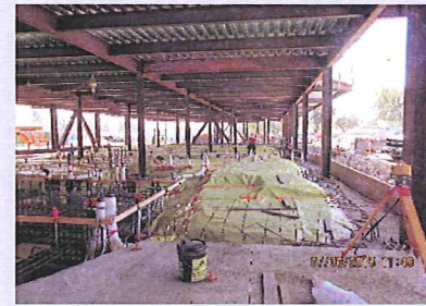
Seg. C -Installation of vapor barrier and rebar for concrete pour at 1st floor
