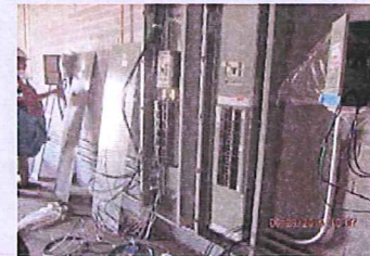
Electrical Panel Wiring
