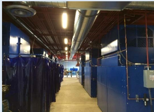
Welding Booths Lab 121
