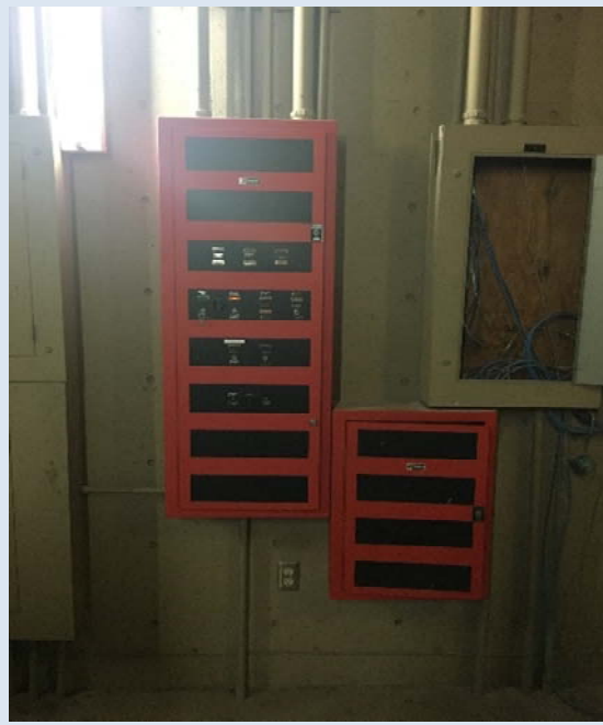
Existing Fire Alarm Panel
