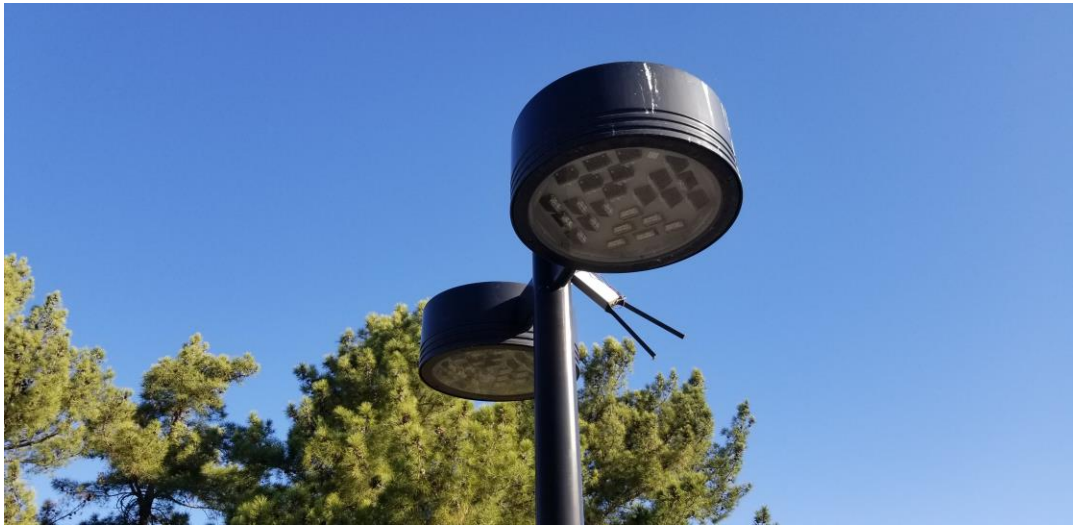
Existing Dual-Head Pole Top – A2
