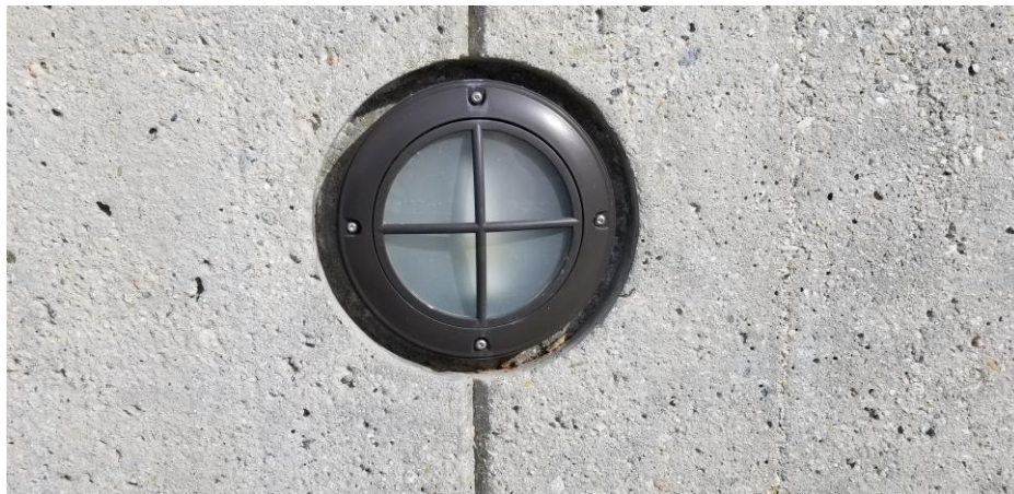
Existing Step Light – S1
